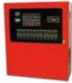
Electronic Fire Alarm Panel
